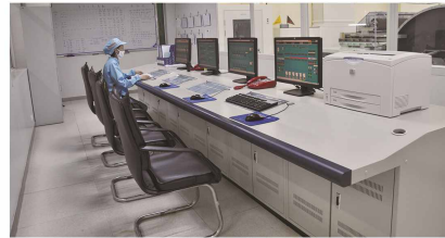
DCS在线监控系统 The DCS Online Monitoring System
