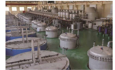
溶液设备 Solution Equipment
